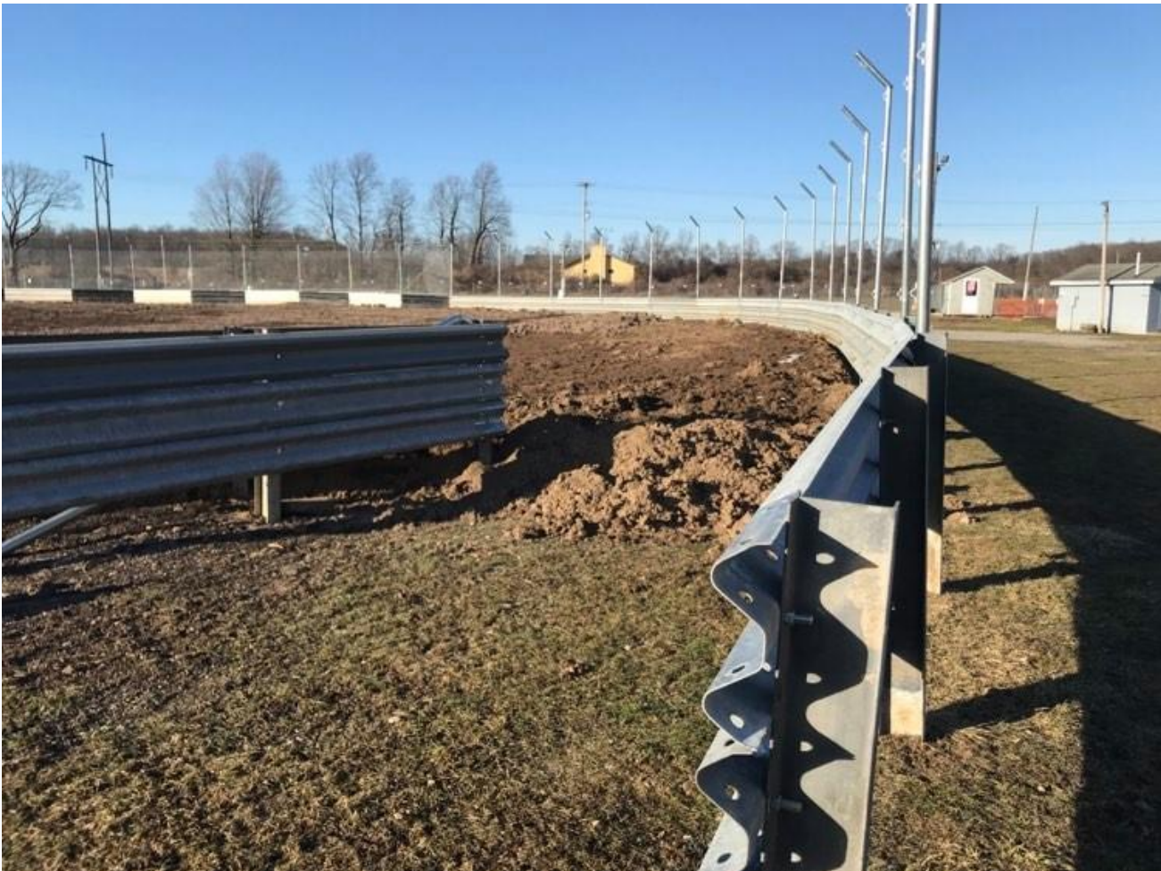
3/8/20 – Installation of new guardrail lining turns 1 & 2 and the track exit to Victory Lane. Soon we will install our fencing.
